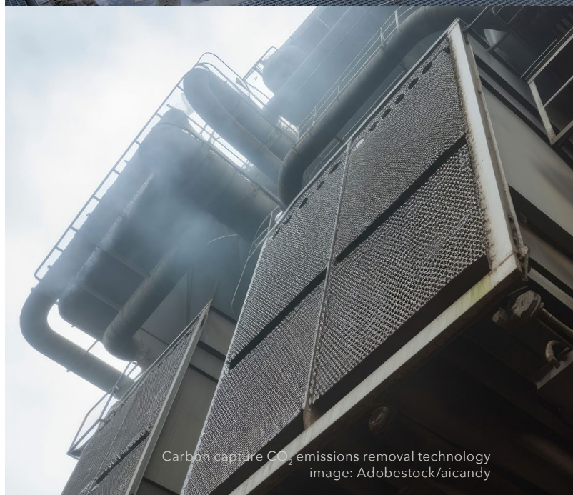
Heat exchanger on the roof of a factory image: Adobestock/geoki
